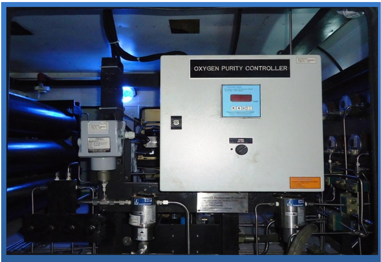
OXYGEN PURITY CONTROLLER PANEL
