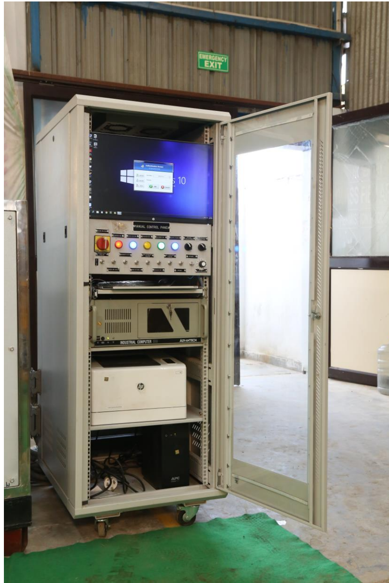
Figure 2: DAQ PANEL FOR DV TEST BENCH
