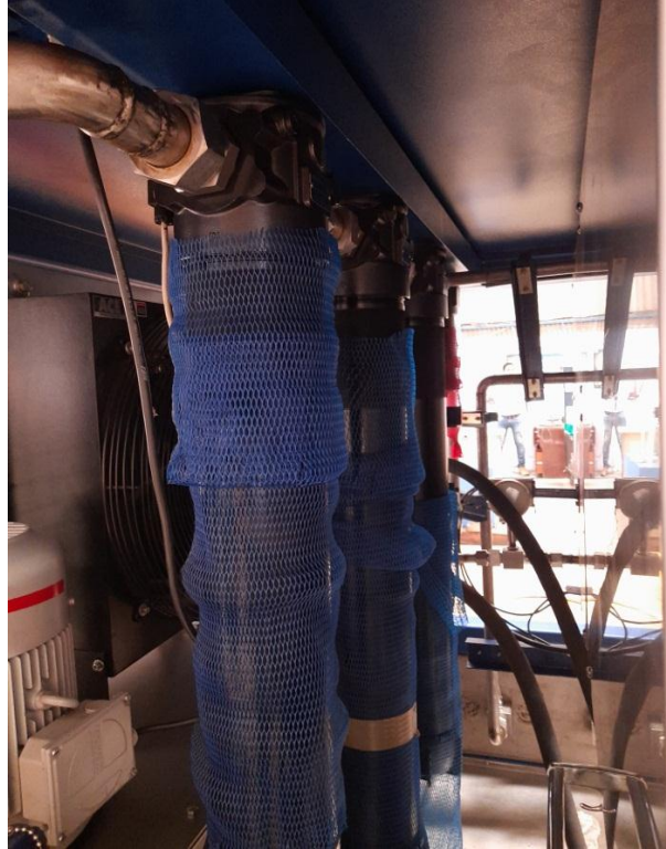
Booster line filter
