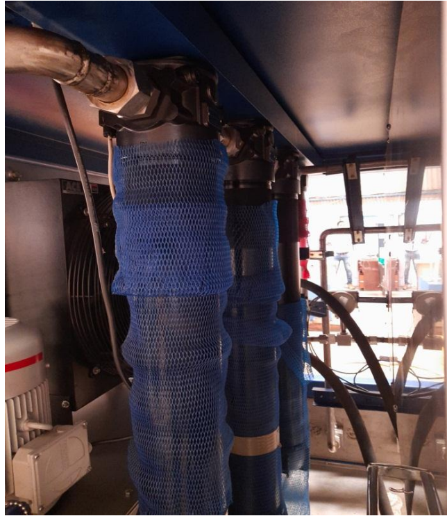
Booster line filter
