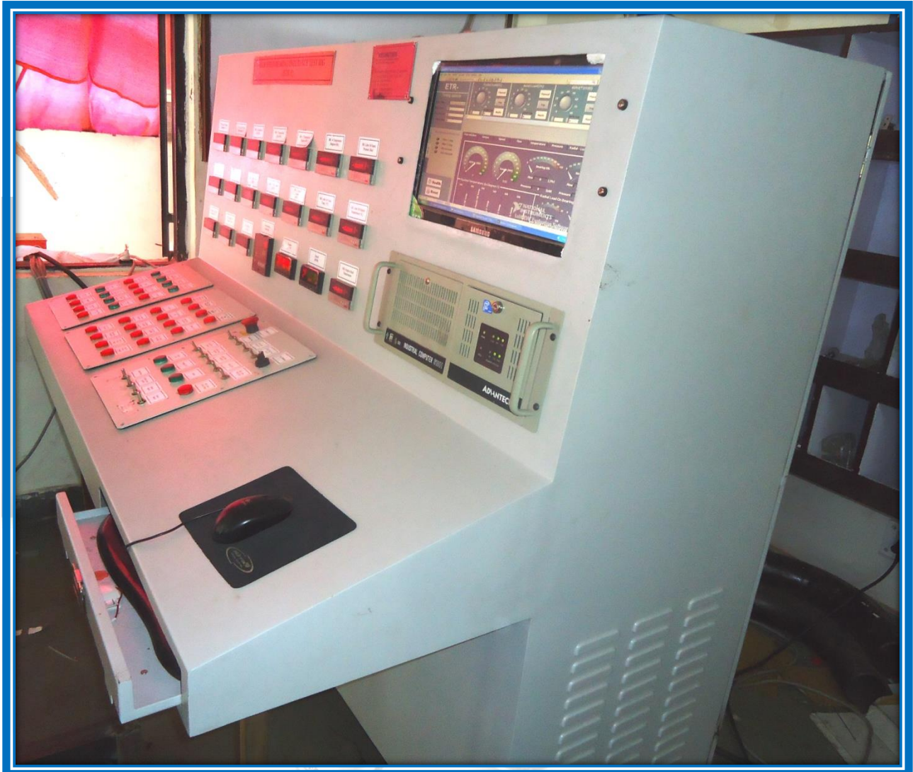
Main operating Panel
