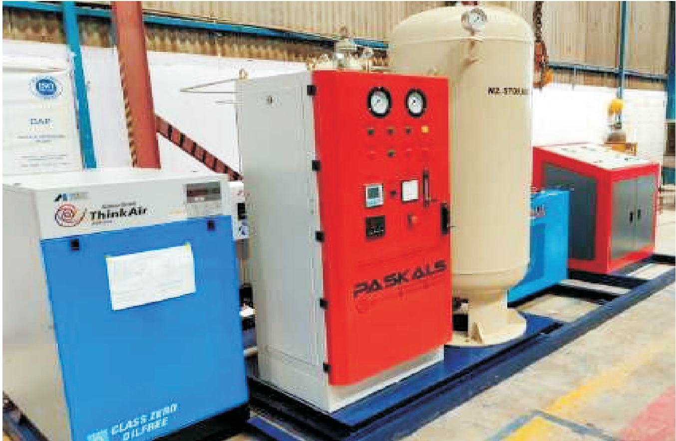
Nitrogen Generation Plant, 99.5% purity, Membrane type, Max Working Pressure 350 bar
