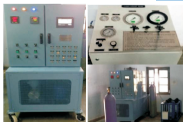
HALON Recovery, Reclamation, Recycling & Refilling Facility
