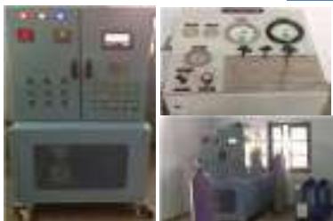
HALON Recovery, Reclamation, Recycling & Refilling Facility
